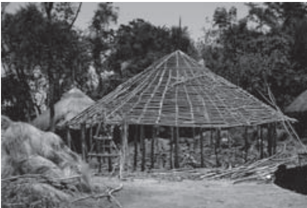
Figure 4. A Luo house ( ot ) under construction, with materials gathered for the project.
