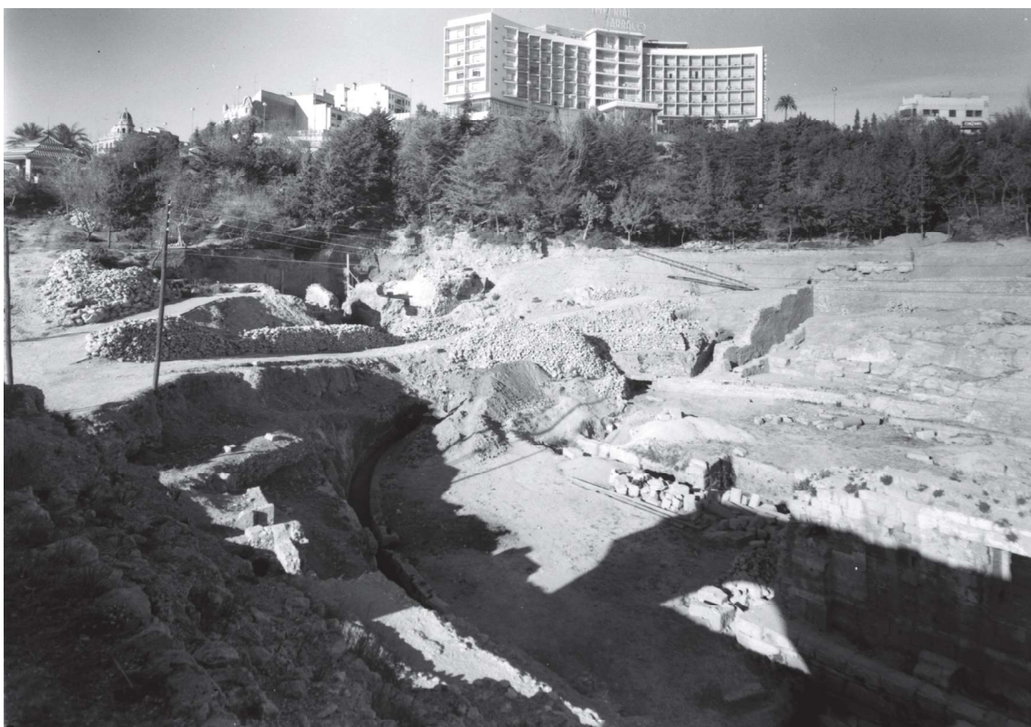
Figure 3. Initial stages of the works directed by Alejandro Ferrant. Northwest view of the complex, from de top of the meridional grandstands. Ferrant archive of the Col·legi d'Arquitectes de Catalunya (COAC), negative catalogued with the number 51_001. Also exist a copy on paper at the AAFV dated januray 26, 1968.
