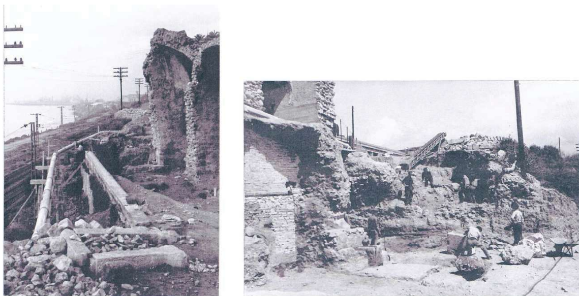
Figure 5. Two photographs of the seaside façade of the southern grandstands. At left dated february 29, 1964; at right april 16, 1964 (AAFV, uncatalogued images).
